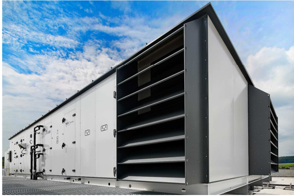
The FFT head office in Fulda is equipped with complete TROX products and systems that provide high levels of comfort, safety and energy efficiency.
