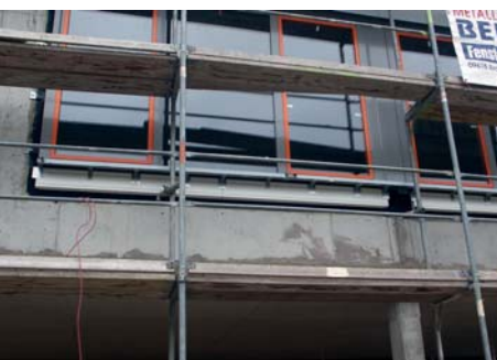
The renovation of the facades of public buildings with thermal insulation is at the top of the list of priorities of German communities.
