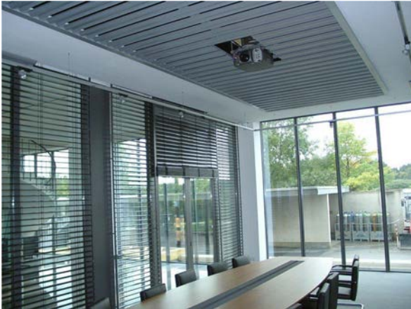
Installation example: Fritzmeier, Germany
