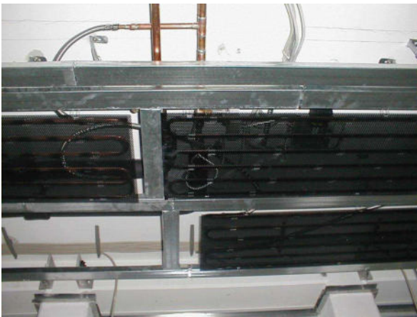
WK-D-GK suspended in on-site support structure
